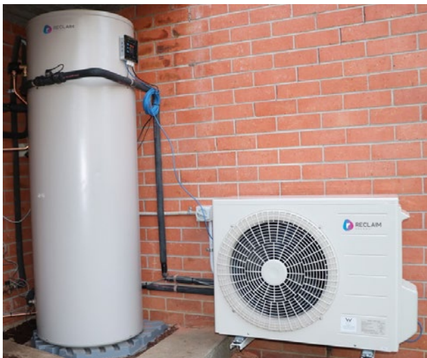
Figure 7: A photo of installed hot water system with proper insulation of pipelines.
