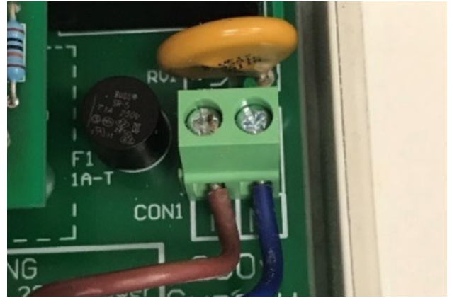
Figure 20: Prewired power cable on terminal block 1 (CON1).
